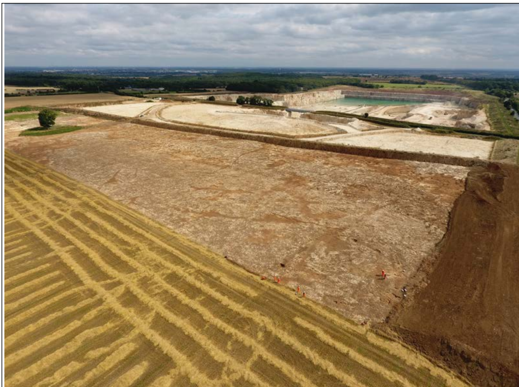
Fig. 5.7. Aerial view of the east part of field N2/N3 after topsoil stripping in 2021, looking north-east.
