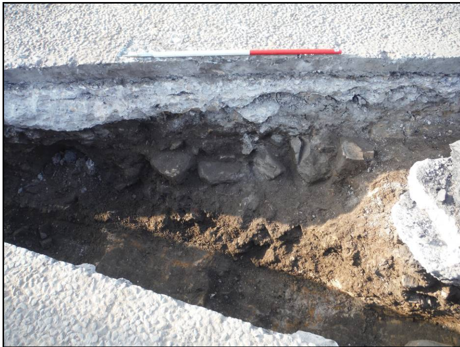
Figure 12. North-west facing section of Trench 2. Note the demolition deposit underlying the concrete road sub-base containing frequent sub-angular sandstone blocks (403). (Scale = 0.5m graduations).
